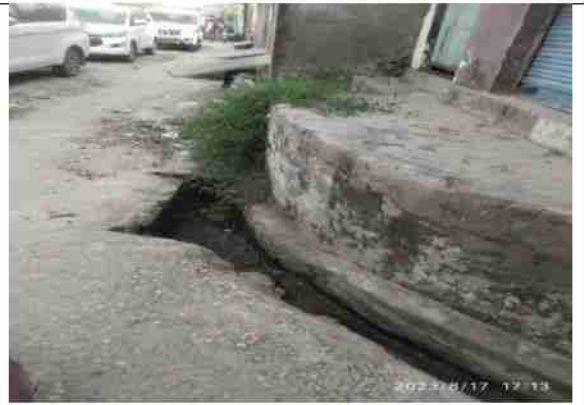
Photo 22: Channel carrying sewage of nirana village to Pond at Khasra No. 333
