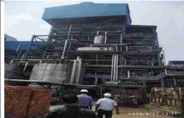
Photo 4: Incineration boiler (60 TPH)
