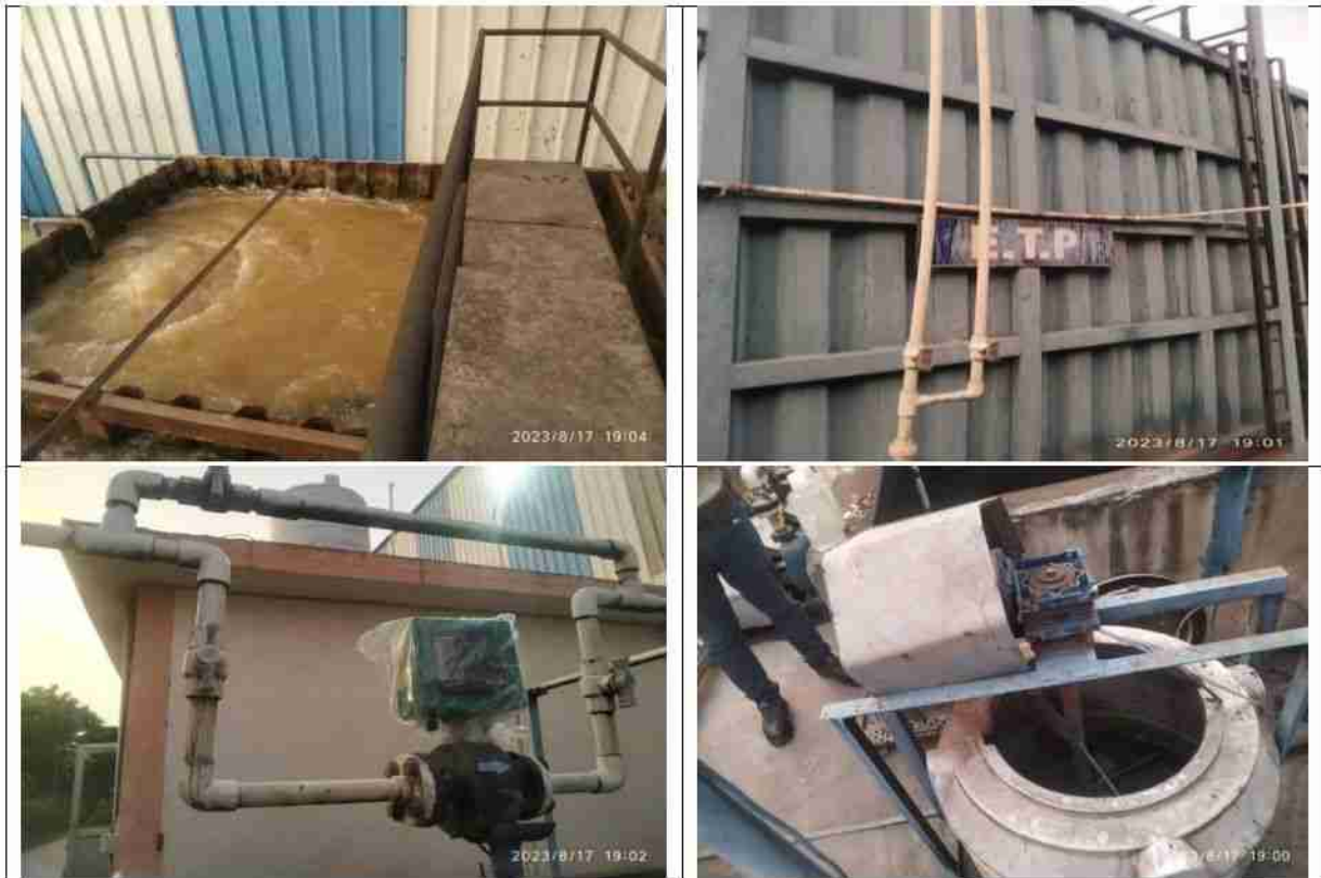
Photo 17: Photographs of ETP at bottling plant
