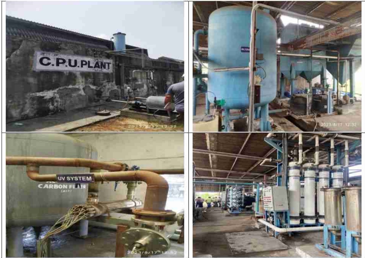
Photo 7: Photographs of CPU installed in Molasses plant
